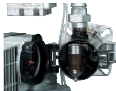
Inspection of combustion head
